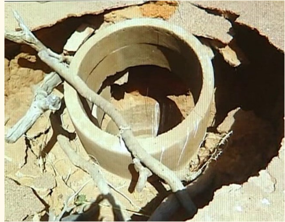
Water point in poor condition
